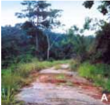
Picture 'A' shows a broken road surface. Mines are often concealed in the potholes. They may also be concealed under the thin tar by melting areas and putting the soft tar back on top of mines.
